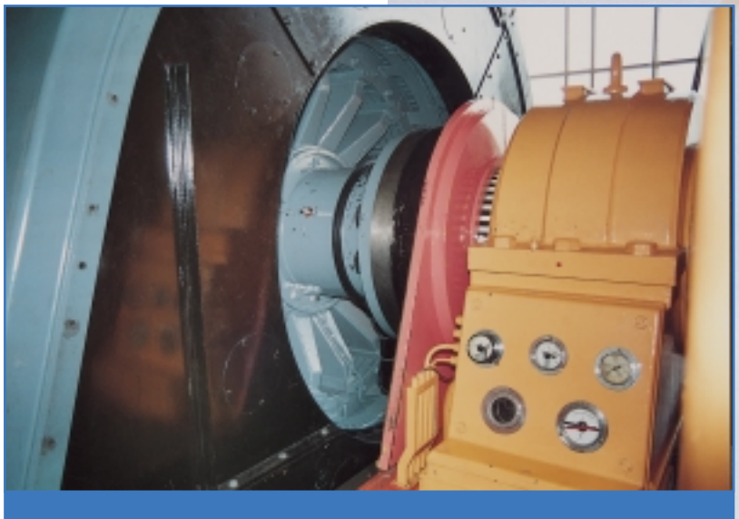
Rotor temperature monitoring on GTO-controlled 50-megawatt motor
